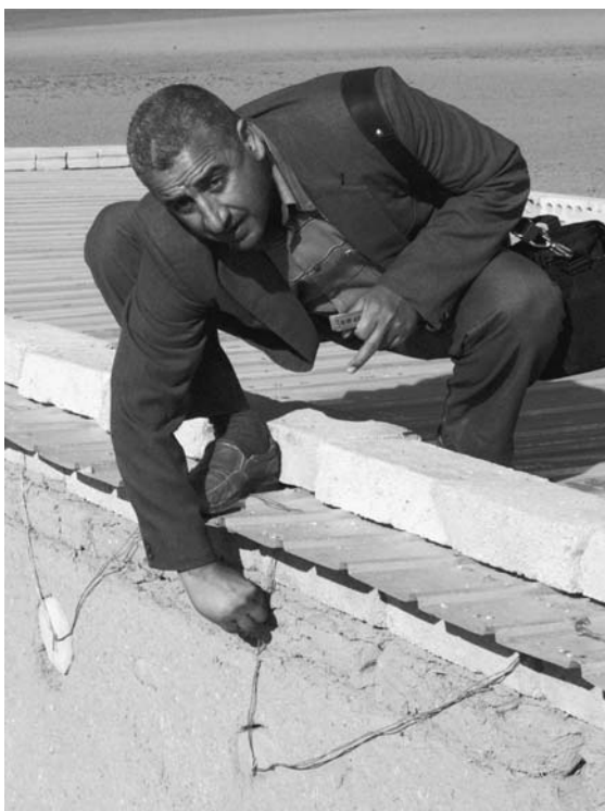
Figure 2. AT LAST, A ROOF TO LAST: Mahmoud “Abu Turki” el-Kitab, majordomo of Hamoukar expedition house, examines repairs of new roof over Hamoukar’s dig house, following five months of winter rain (April 2005)
