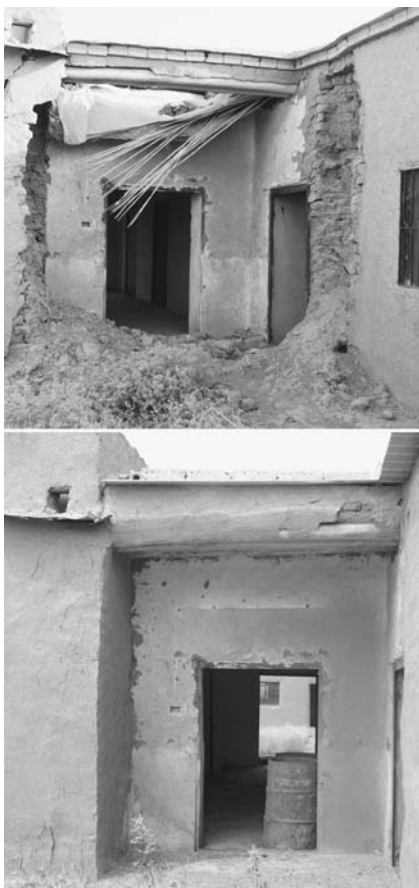
Figure 4. REFURBISH AND RESTORE: Passageway between inner and outer courtyard of the dig house, bathrooms on the right side, entrance to dining room area visible in passage way; (above) water damage to roof and partial wall collapse (October 2004), (below) same area following basic repair to walls and roof, before replastering of alcove (April 2005)
