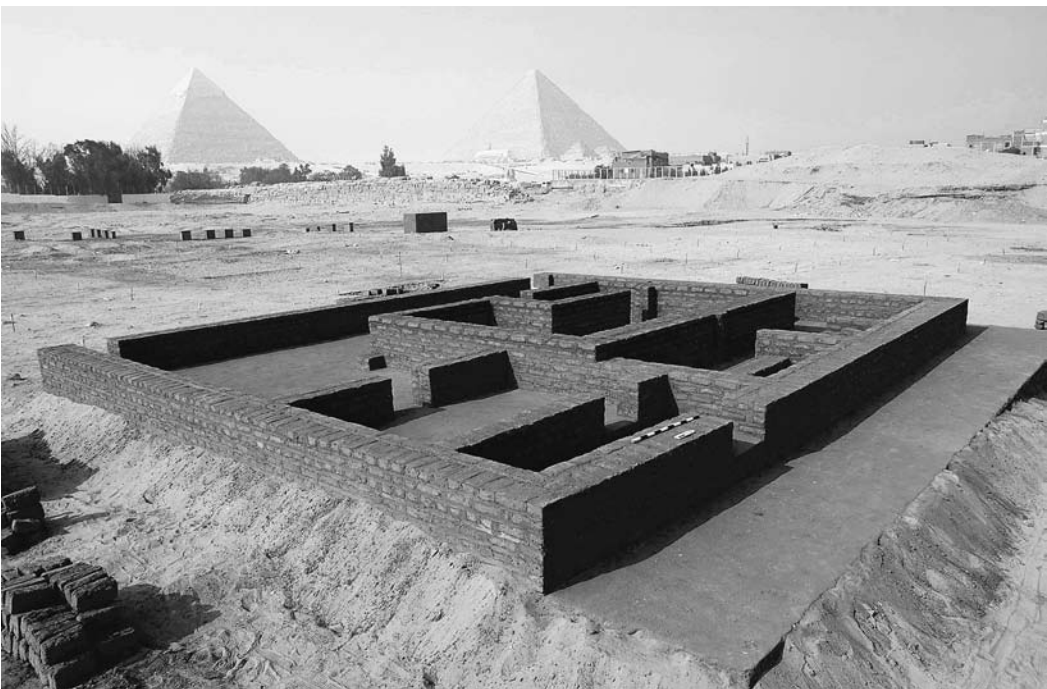
Figure 13. The completed reconstruction of the Eastern Town House built on top of a thick layer of sand over the ancient house. View to the northwest
