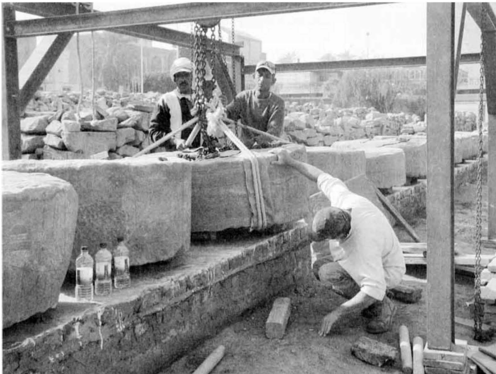
Sayid, Ali, and Dany lifting column drums onto protected platforms, Luxor Temple
