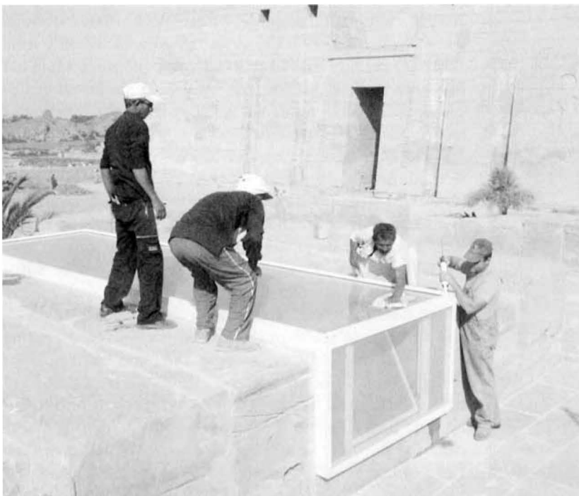
Ali, Sayid, Hassan, and Dany installing the skylight, small Amun temple, Medinet Habu
