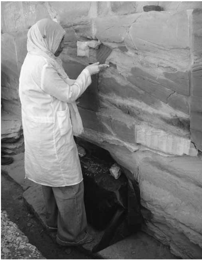
Conservator Hala consolidating the back wall of the small Amun temple sanctuary
