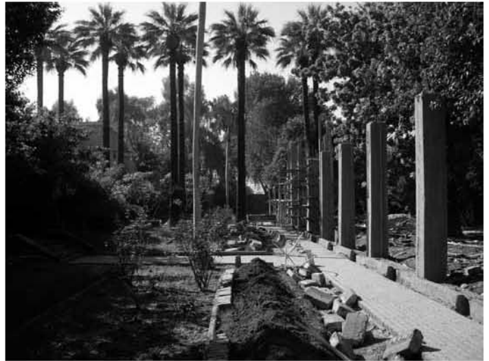
The Chicago House front garden wall going up, December 12, 2008. Photo by Ray Johnson
