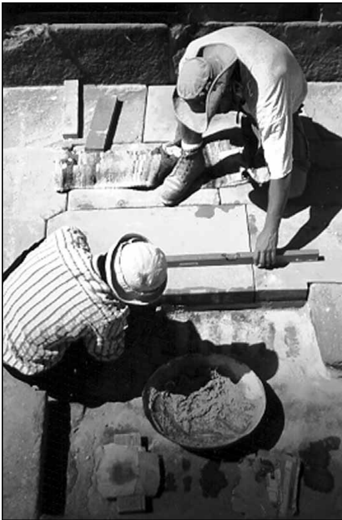
Dany Roy supervises restoration of Ptolemaic roof blocks. Small Amun Temple, Medinet Habu, 1998/99 season. Photograph by W. Raymond Johnson
