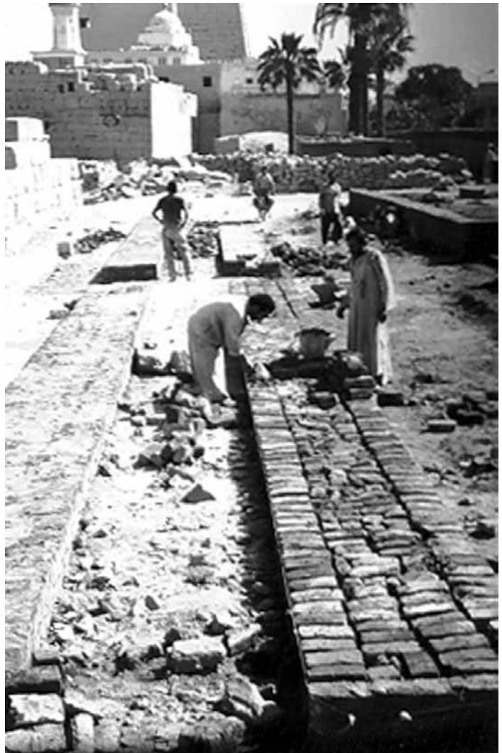
New storage platform under construction. Luxor Temple, Epigraphic Survey blockyard, 1999. Photograph by W. Raymond Johnson
