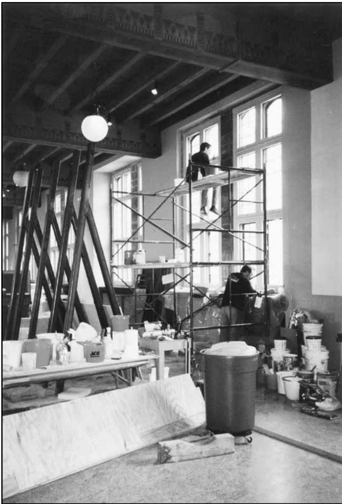
Figure 4. Nathaniel Ward of Ars Artis Restoration works with assistant cleaning and repairing stone walls in north gallery
